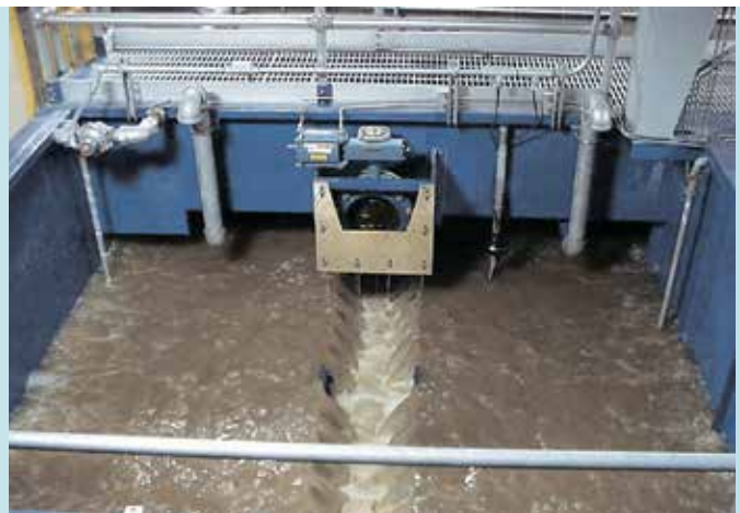
Backwash water flowing in trough, air assisted
