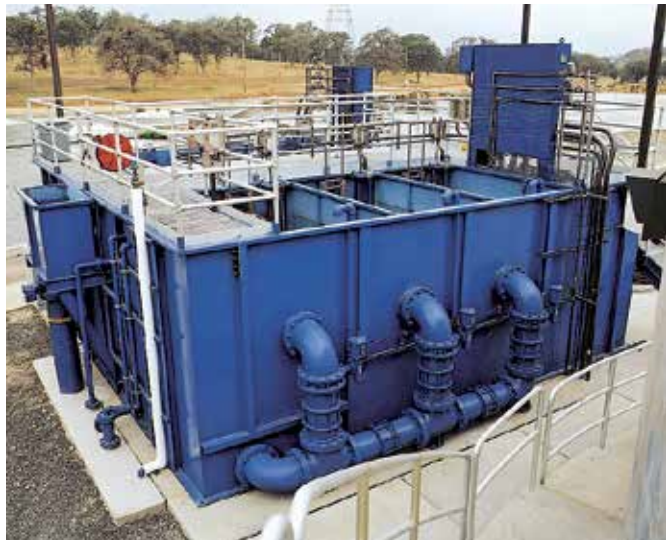
The Chem-Clean® system restores the sand to its original condition.
