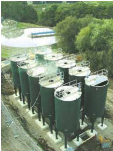
Municipal wastewater polishing application for ammonia, BOD, and suspended solids removal.
