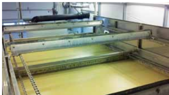
Top view of DGF providing phosphorous removal.
