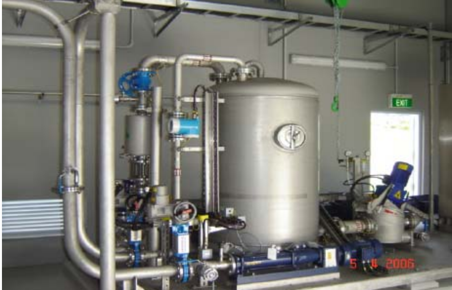
Figure 5. Crown™ Disintegration System at Rosedale WWTP, North Shore, NZ.
