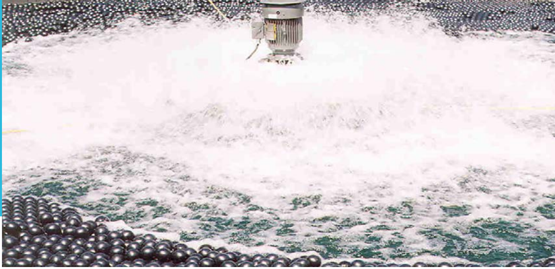
Aqua-Lator® Surface Aerator installed with E-Ball® Floating Cover System
