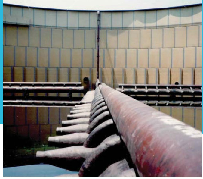
VARI-CANT® Jet Mixing System installed in circular basin.
