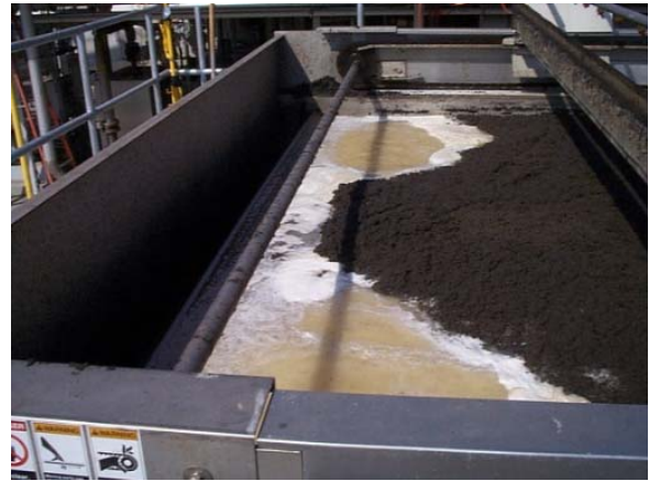
Figure 3. DAF clarifier with same bulking activated sludge
