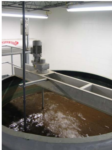
Figure 7. Aerated tank effluent in flocculation tank prior to DAF
