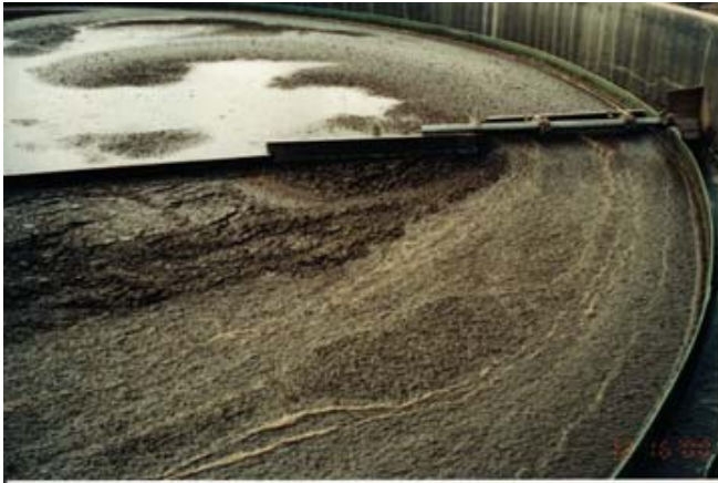
Figure 2. Gravity clarifier with bulking activated sludge
