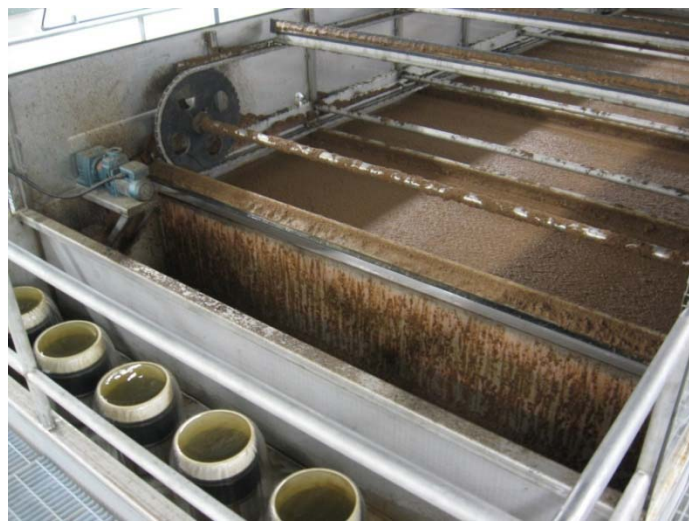
Figure 8. DAF providing clarification of aerated tank effluent
