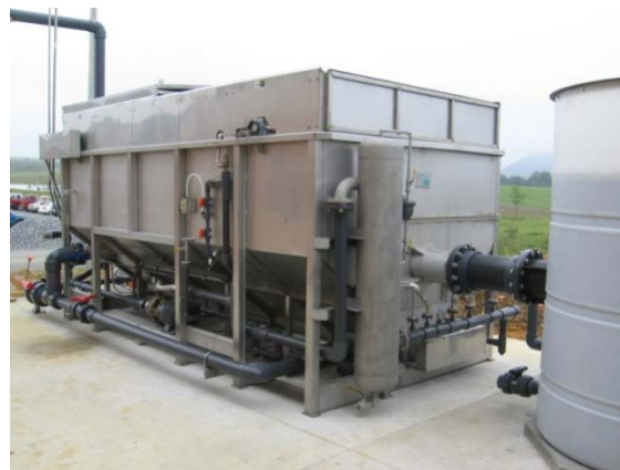
Figure 6. DAF clarifier with flocculation tank treating anaerobic effluent
