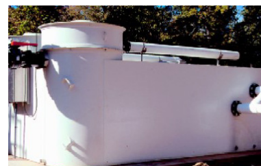
Deep-Bed Sand Filters
