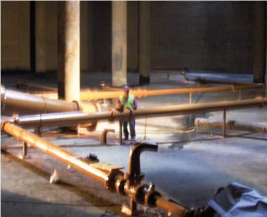
JetMix system installed at MMSD South Shore WWTP
