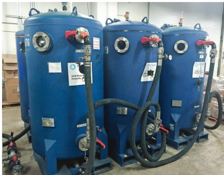
Wastewater ion exchange tanks for final metal polishing.
